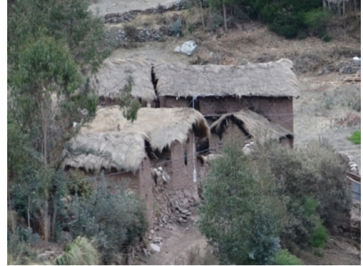
Figure 2. Vulnerable houses in Huaró. (Credits: Centro Tierra).
