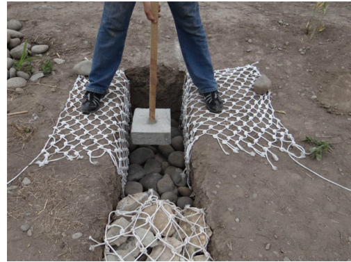
Figure 4. Field test of shicras foundation system to avoid use of clay and to stop water raising into the walls (capillarity). (Credits: Centro Tierra).
