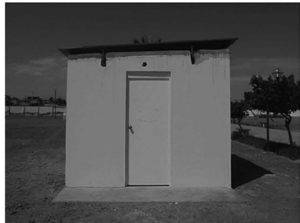
Figure 6: View of the concrete block module with galvanized corrugated steel sheet over ventilated structure as roofing.
